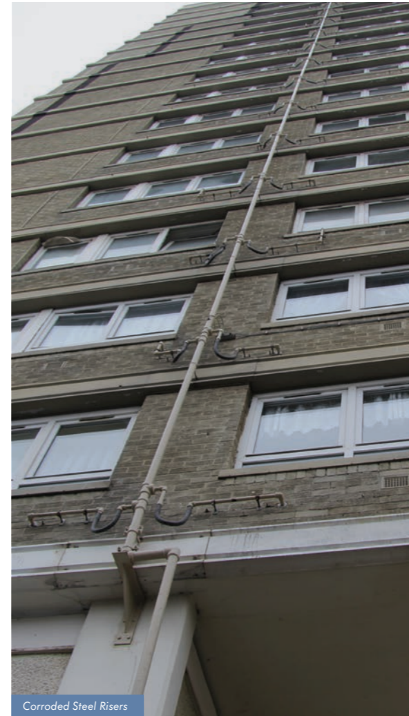
Corroded Steel Risers
